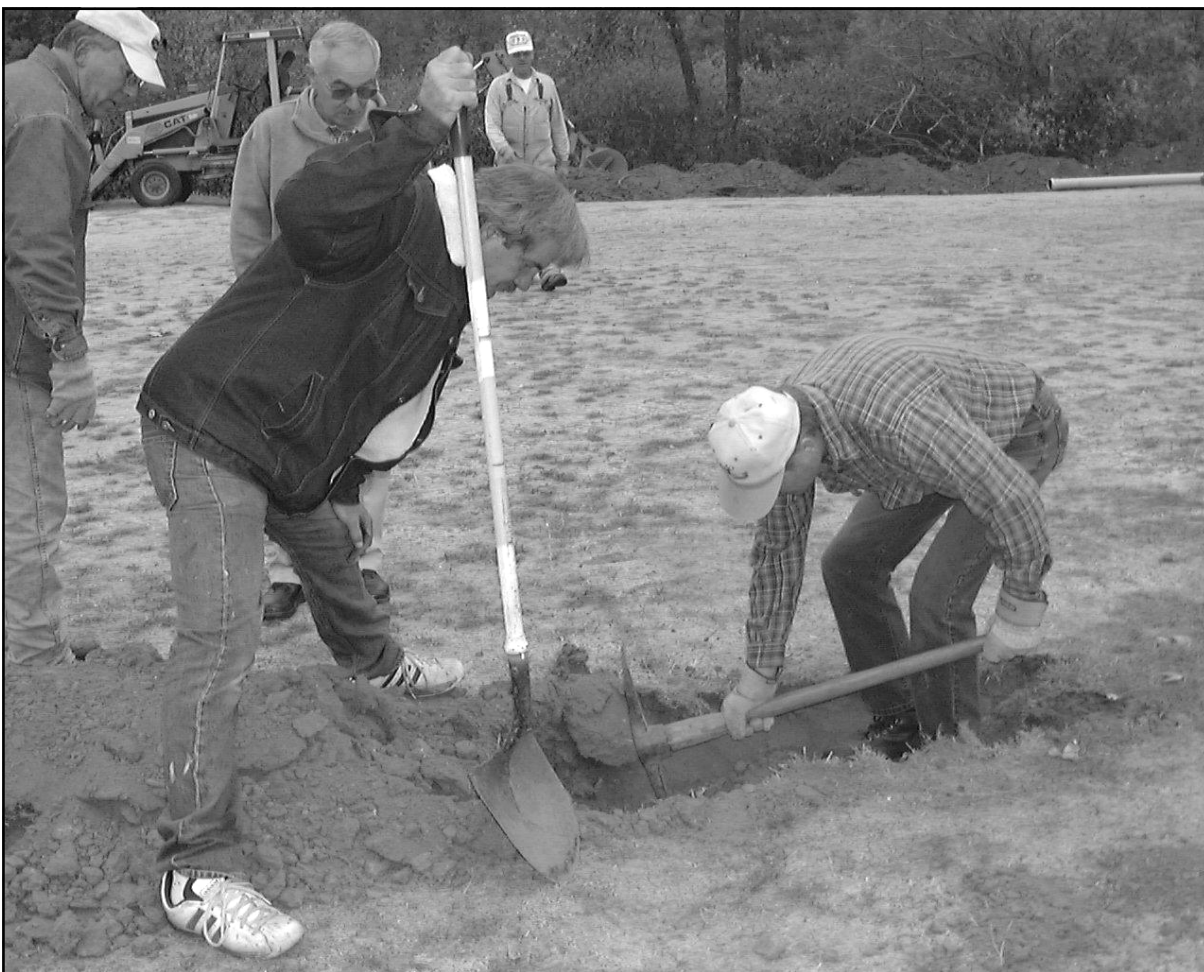
GOLF COURSE WATER - Installation of a 3,000-foot water line at Illinois Valley Golf Course began late last month. The overall project to help supply water for the course will take approximately a month. With a shovel is Bob Hurt and picking along to help is Marv Ahlers. (Photo by Britt Fairchild)
