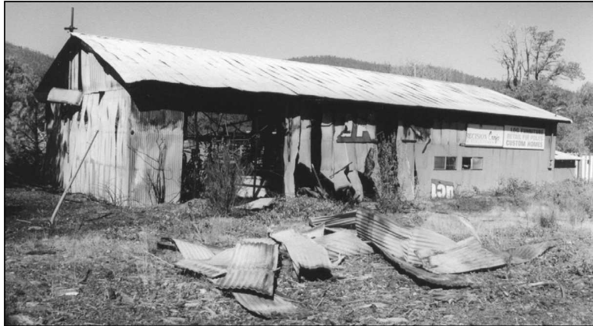
KAUFFMAN WOOD 'RECOVERING' -- Following a two-alarm blaze that began close to midnight on Sunday, Sept. 15, Kauffman Wood Products owner Darrel Kauffman said that his business is working to recover. The loss to the building, owned by Bill Pfohl, and the contents, owned by Kauffman, was estimated by Illinois Valley Fire District at $200,000. Kauffman said this week that insurance will cover $35,000 of the loss. "We're reeling and rocking, but keeping on with a smile, and striving to keep producing," said Kauffman. The building might be replaced by Pfohl. Cause of the fire hasn't been determined; Kauffman suspects wiring.
