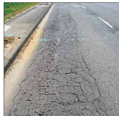
Arterial in poor condition
