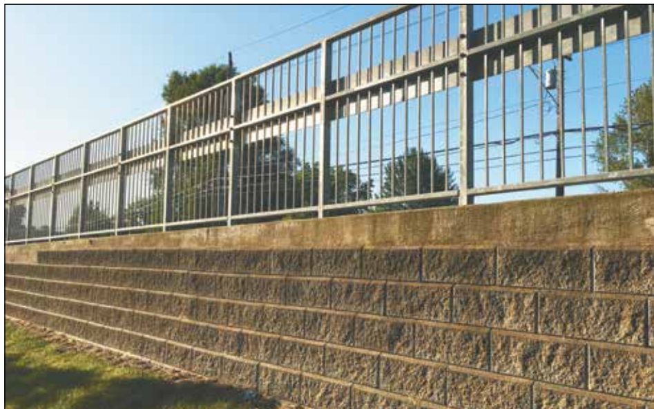
A cast-in-place wall was the design that most residents along Capitol Highway liked. Railings are required where a fall hazard is present. Residents preferred railing that was painted black, which is designed to fade into the landscape. (Post photo by Erik Vidstrand)
