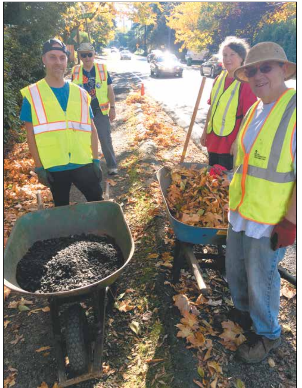
Gravel was delivered by the Portland Bureau of Transportation for the "goat path" along Southwest Capitol Highway on Oct. 28. Volunteers Josh Byler, Donna Jean Paterson, and Chris Houghton use wheelbarrows to spread out the gravel and then tamp it down. Don Baack of SW Trails organized the event. Nearly two dozen neighbors helped out on the brilliant autumn day. (Post photo by Erik Vidstrand)
