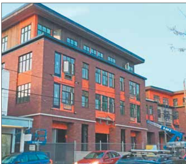
Bremik Construction expects to complete the Multnomah Village Apartments by late fall. (Post photo by Erik Vidstrand)
