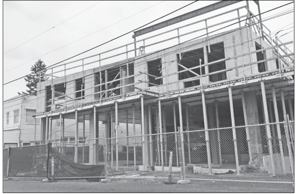
One infill project that has the land use committee concerned is the 70-unit, four-story apartment building under construction on Southwest Capitol Highway at 33rd Avenue in Multnomah Village. (Post photo by Erik Vidstrand)
