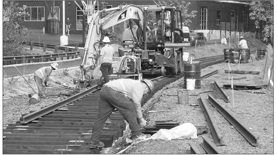
Laying track for the trolley line south of Freeman Motors. (Photo courtesy of Multnomah County)
