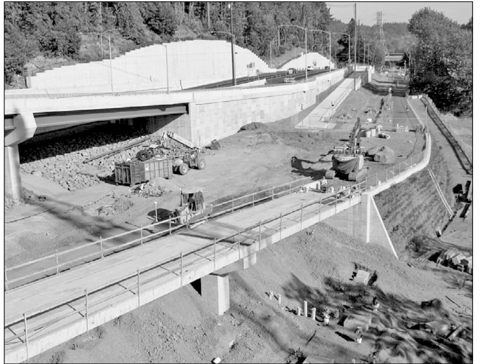
The lower bridge will carry bicyclists and pedestrians from the westside trail to the south side of the Sellwood Bridge. (Photo courtesy of Multnomah County)
