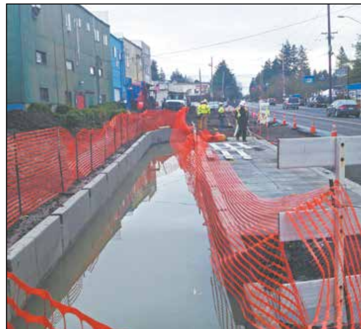
Workers complete construction on a new catch basin and sidewalks along Multnomah Boulevard near 36th Avenue. (Post photo by Erik Vidstrand)
