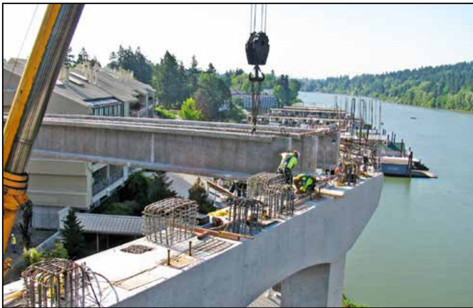
Workers install girders on Bent 6 on the east side approach of the new Sellwood Bridge. (Photo courtesy of Mike Pullen, Multnomah County)
