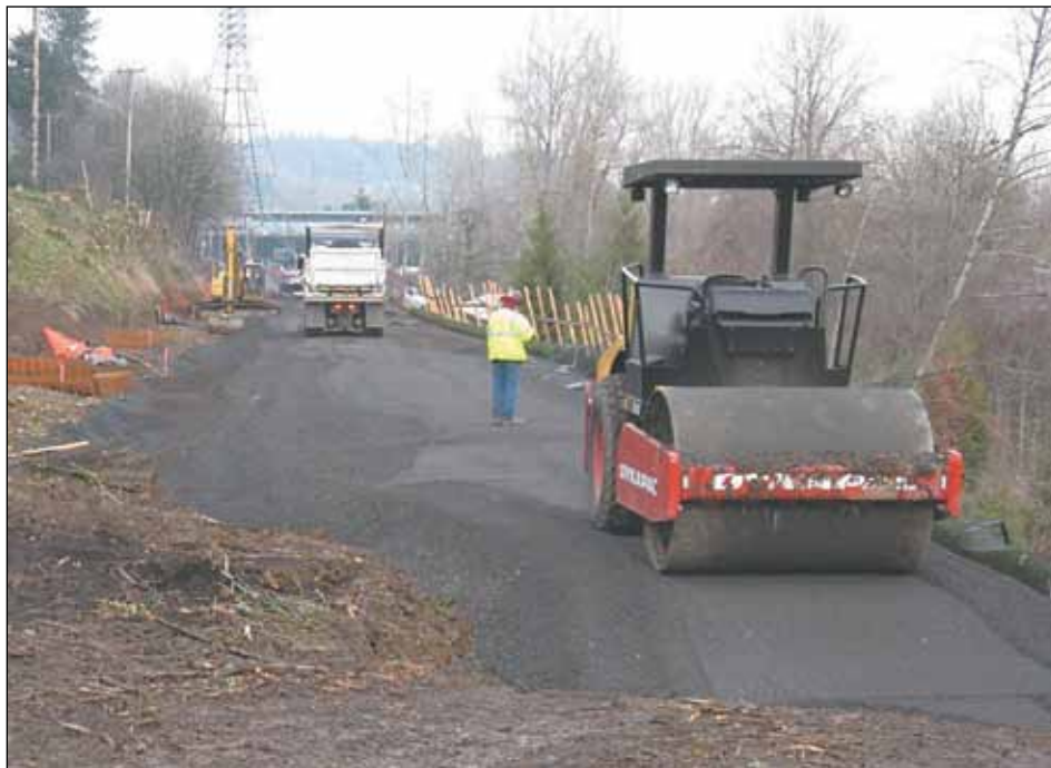
Sellwood Bridge workers pave the new trolley corridor on the west side of the Willamette River in early January. (Photo courtesy of Multnomah County)
