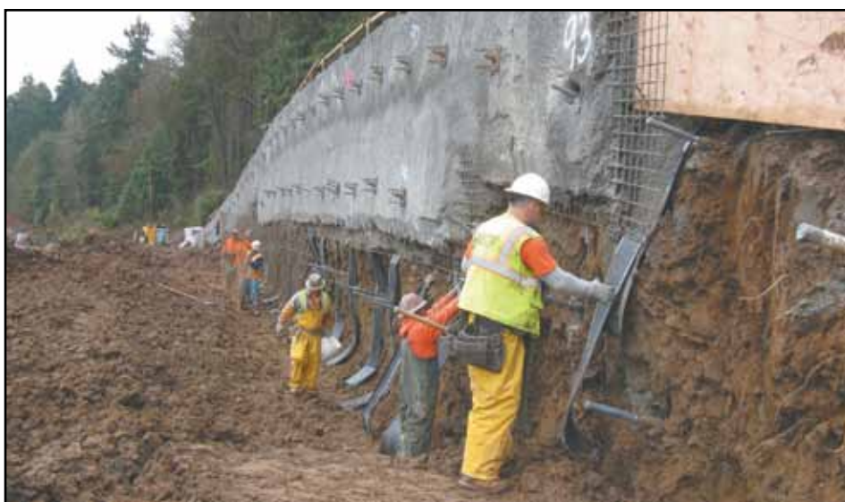
The contractor continues to install soldier piles, soil nails, drainage and shotcrete on the retaining walls north and south of the Sellwood Bridge. Macadam Avenue (Highway 43) traffic lanes will shift west along the new walls in January.
