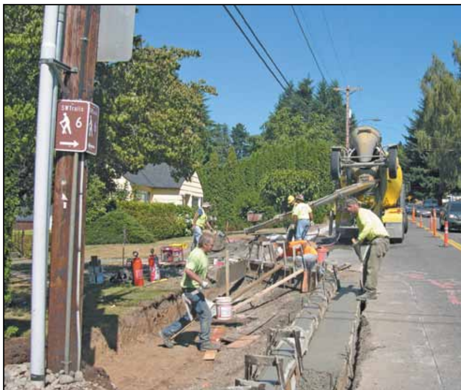
Construction workers pour cement on the new sidewalks along Southwest Sunset Boulevard at DeWitt Street, July 26. (Post photo by Don Snedecor)
