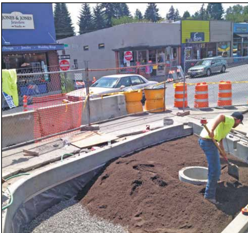
A city contractor works on the new bioswale at Southwest 36th and Capitol Highway in front of ZoomCare. (Post photo by Erik Vidstrand)
