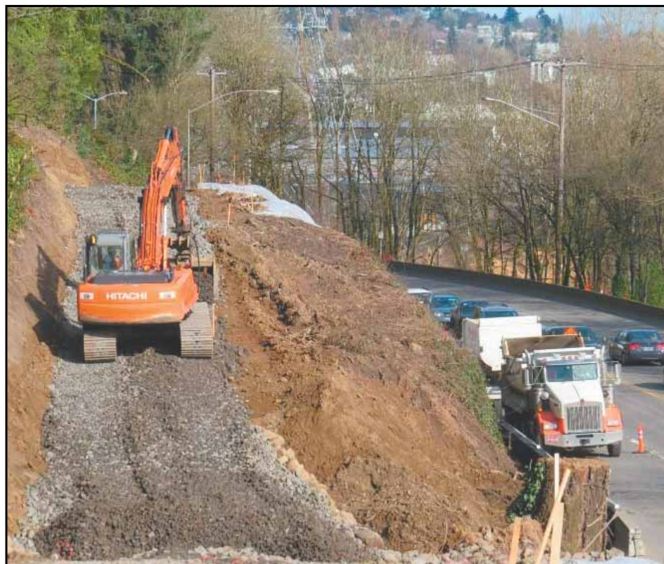
Crews excavate the west side of Highway 43 in preparation for the new Sellwood Bridge. (Photo courtesy of Multnomah County)
