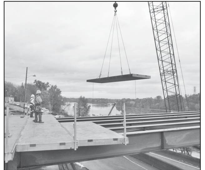
Construction continues on the Sellwood Bridge as workers add deck panels to the west approach of the detour bridge. (Photo courtesy of Mike Pullen, Multnomah County)
