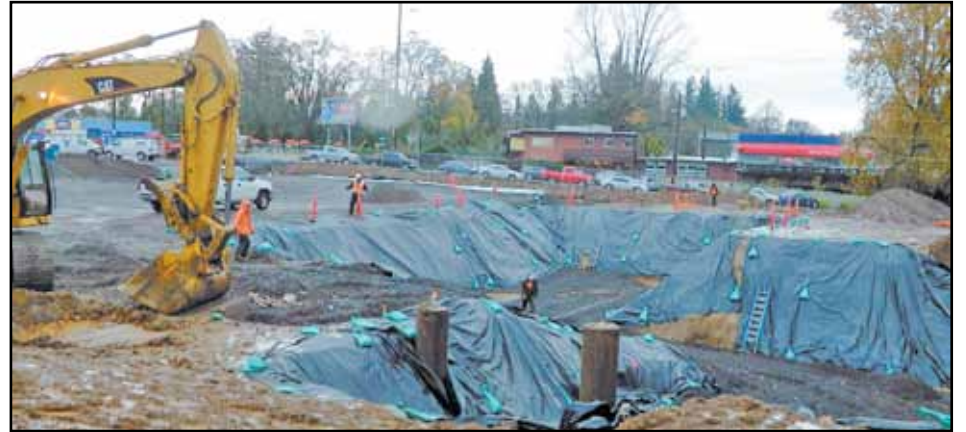
Footings are being installed for the new Safeway under construction at Barbur Boulevard and Capitol Hill Road. (Post photo by Erik Vidstrand)
