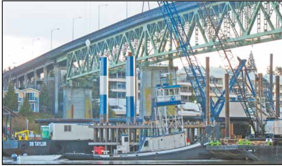
Detour bridge river work being done using a tugboat last month. (Photo courtesy of Mike Pullen, Multnomah County)
