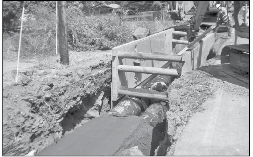
This photo taken July 12, 2010 by a city inspector shows new sewer pipes being installed along Multnomah Boulevard.
