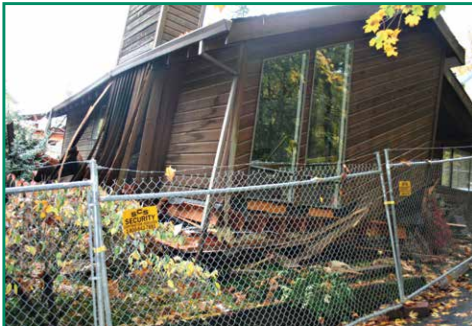
This photo taken on November 9 shows one of the homes damaged in the Terwilliger landslide. (Post photo by Polina Olsen)
