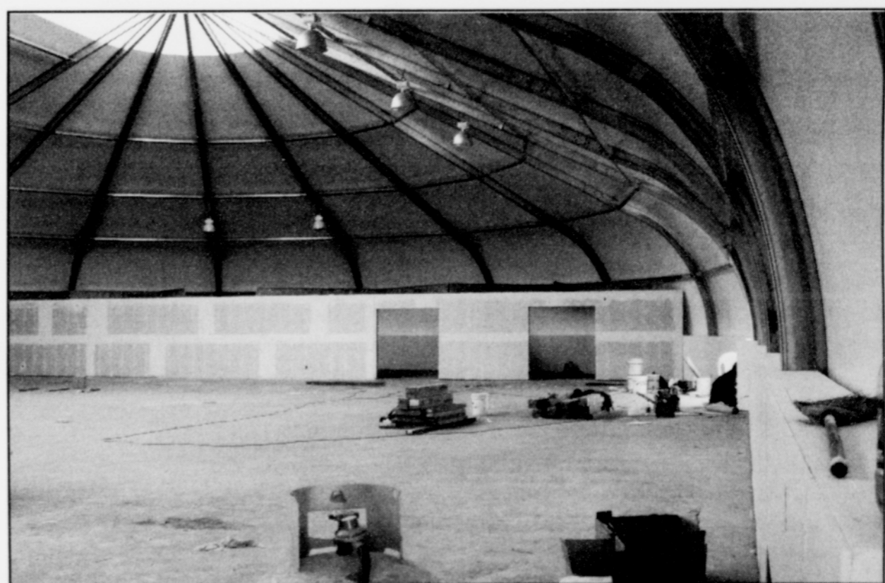
The wrestling room and a storage area are being walled off in the new gym in Siletz. Estimated opening date for the gym is in July. (photo by Diane Rodriguez)
