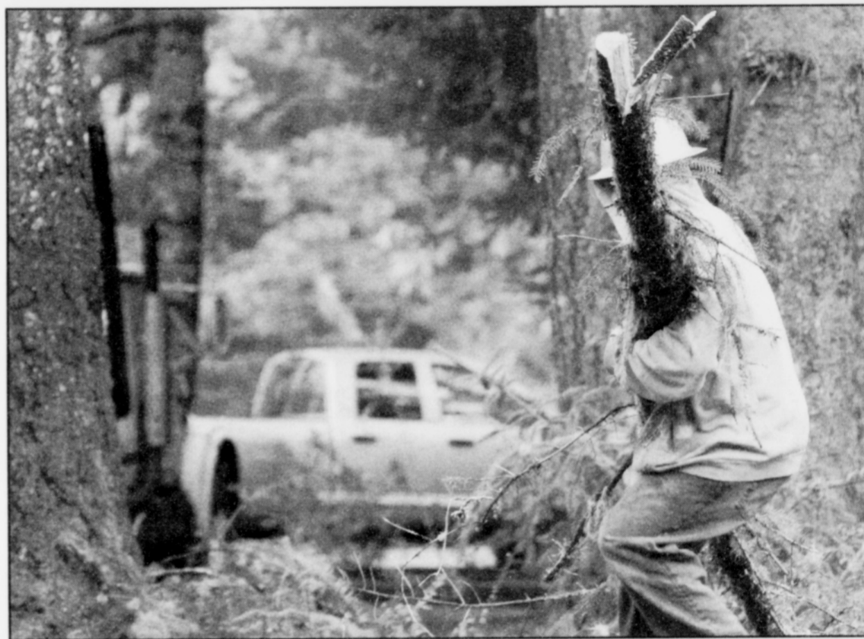
Tristen John helps remove tree limbs in early March as trees are cut down to make room for the cultural repository on Government Hill in Siletz.
