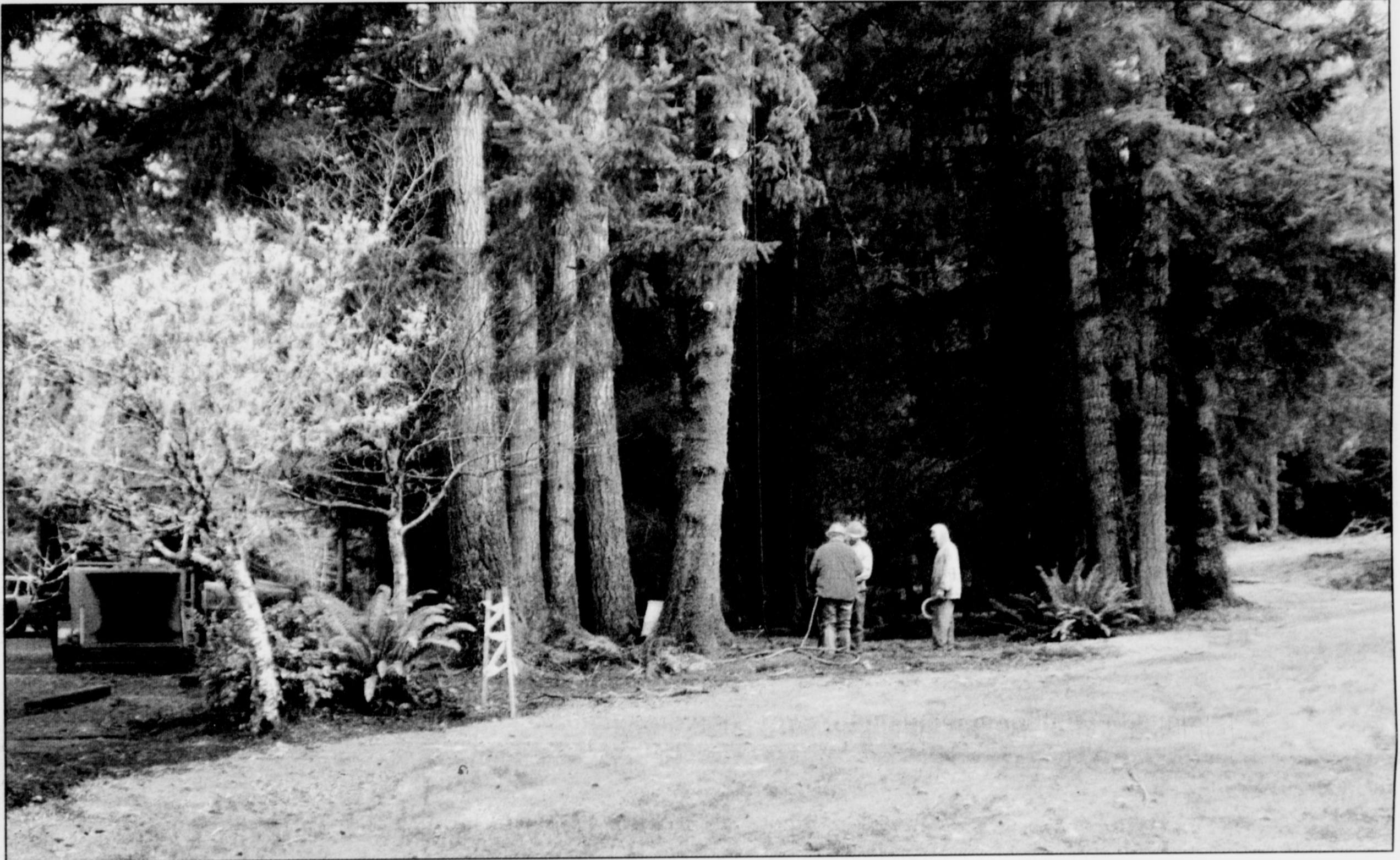
A crew from Busy Beaver Tree Service in Otis, Ore., prepares to cut limbs from trees near the Siletz Tribal Community Center prior to removing the trees so the construction of the cultural repository can begin. As this issue of Siletz News was going to press, the cement foundation for the repository was being poured.
