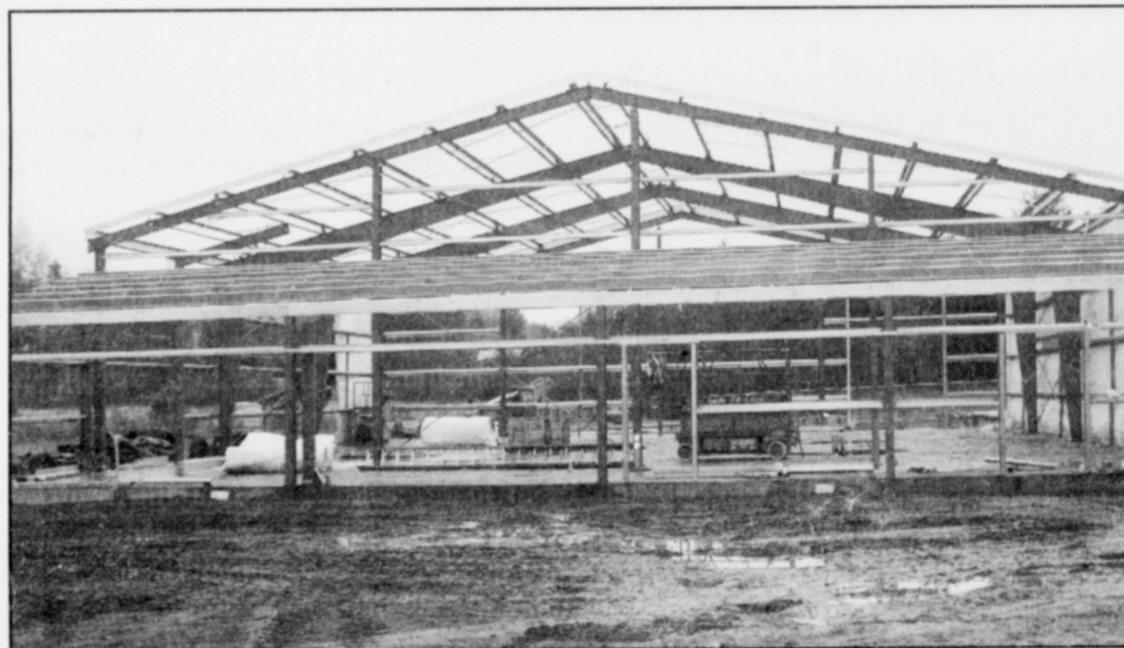
The new USDA building starts to take shape just east of the city of Siletz. (photo by Diane Rodriguez)
