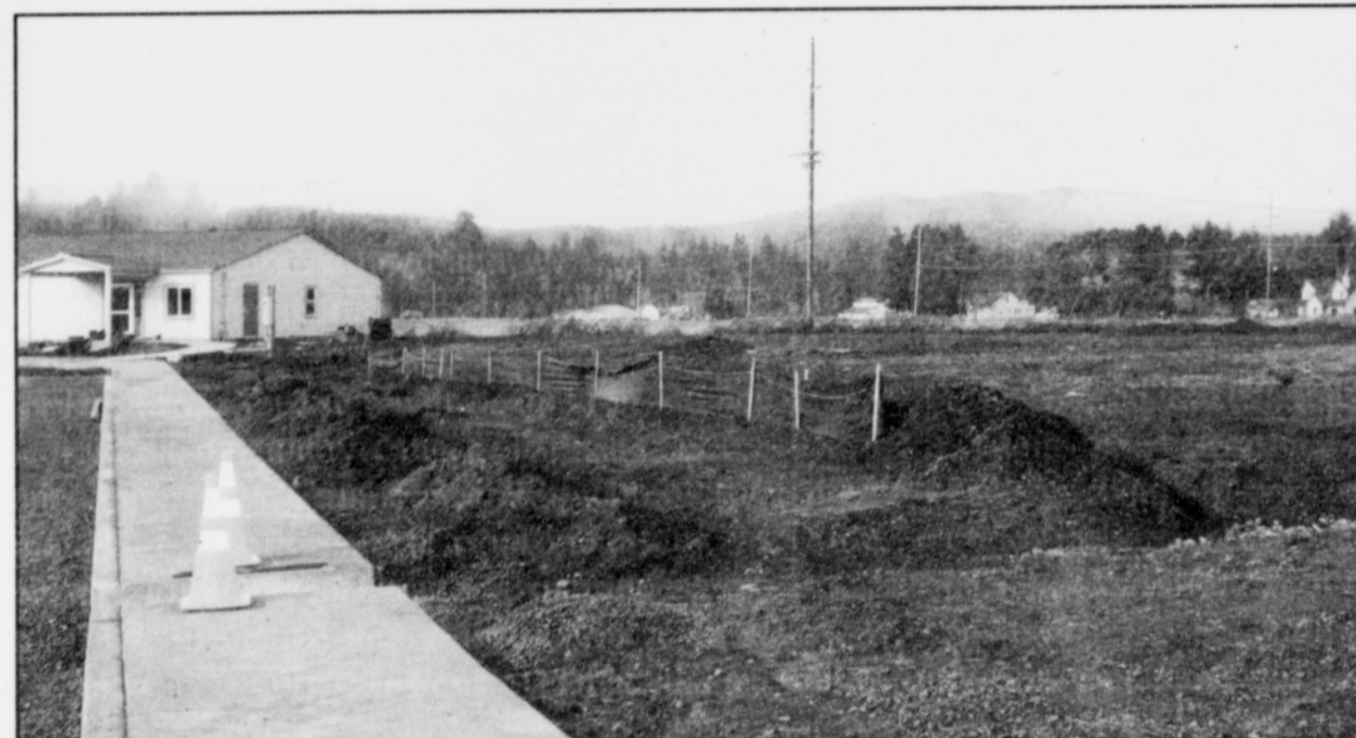
Land for the new gym has been cleared near the Fitness Center building.
