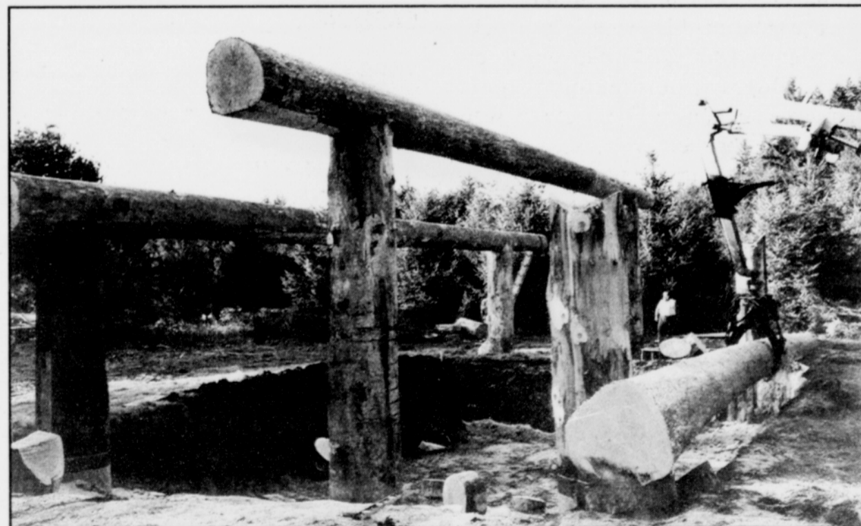
Logs start to outline the frame of the Dance House in the early stages of construction in the mid-1990s.
