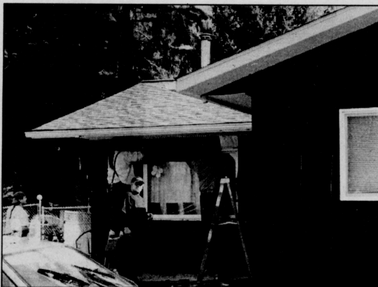
Kevin Goodell's house receives new siding in October. Tribal members were employed to install siding on all the homes up on the hill in Siletz.
