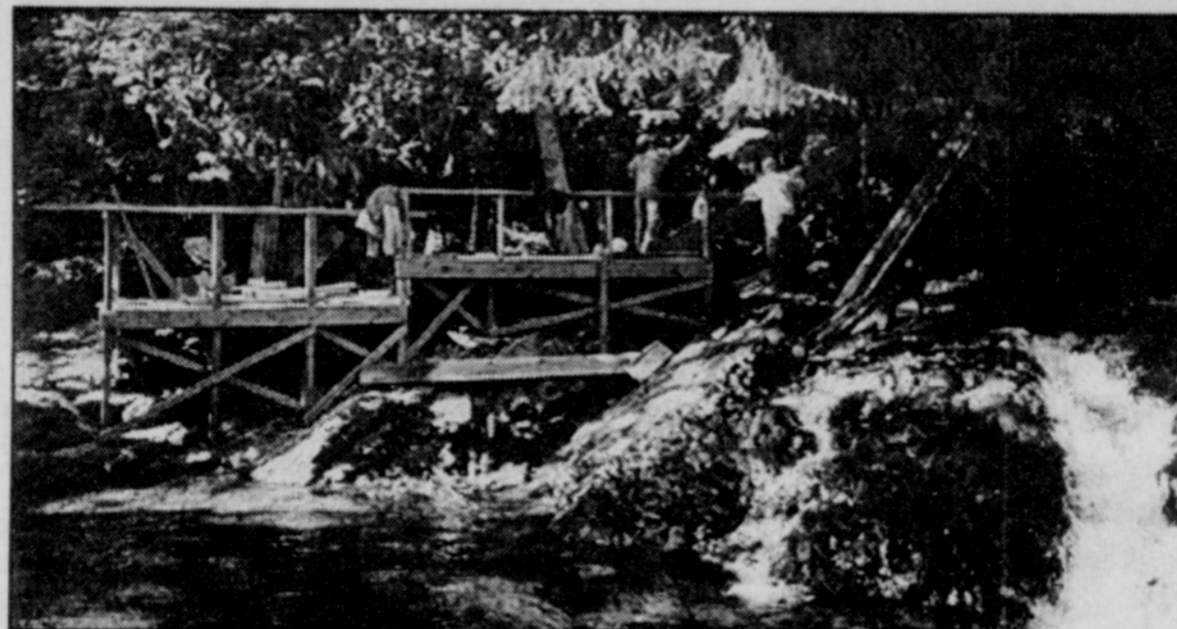
Jay Christensen, Frank Simmons, and Harold McCord are part of the team that worked on replacing the fishing platform at Euchre Creek. See page 15 for the finished product.
