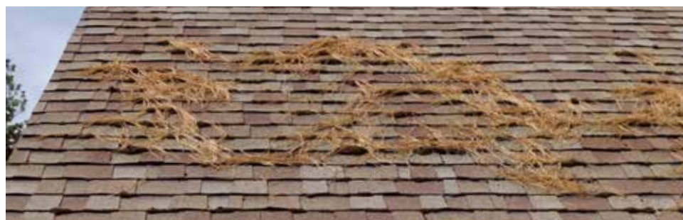
As we head into what could be a severe fire season, homeowners are urged to lessen fire danger by taking such steps as clearing pine needles off their roofs. Photo: Sandy Shaffer.
