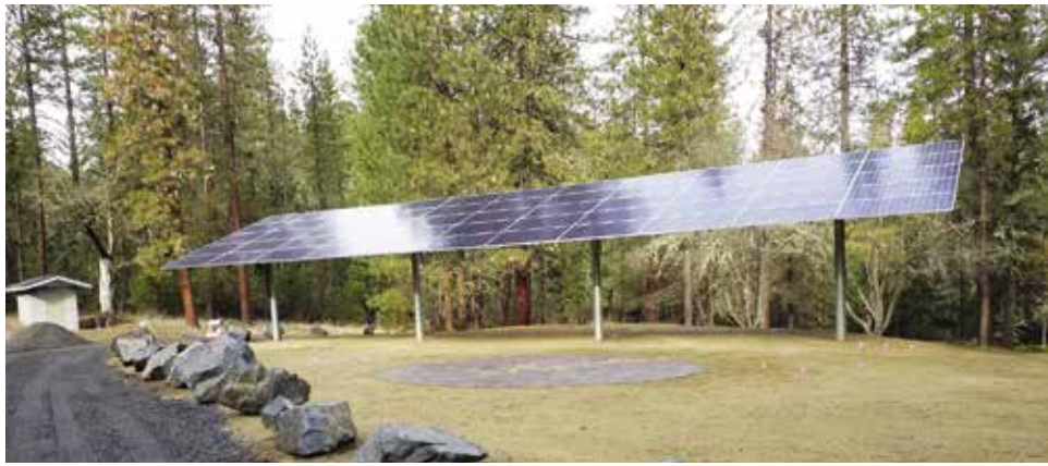
The newly installed solar array at Cantrall Buckley Park. Photo: Cathy Rodgers.
