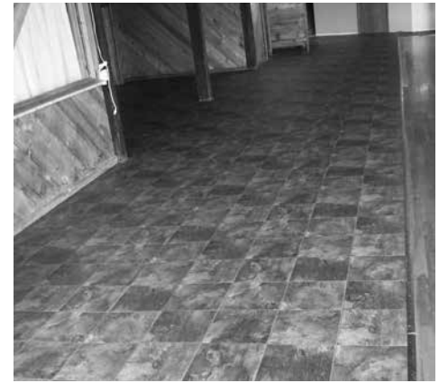
New flooring in the Cedar Center thanks to the Carpenter Foundation, Lippert's Carpet One, and Rodger Miller.
