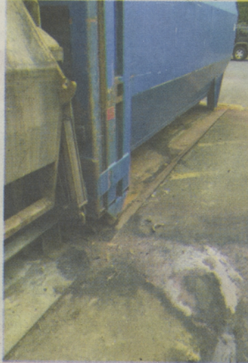
Top: The pictured dumpster was the source of waste leaking into a nearby storm drain behind the Community Center.
