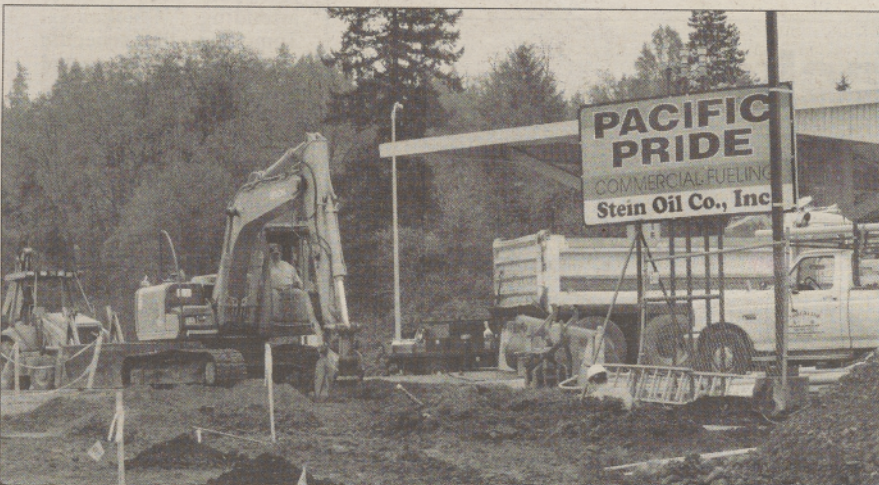
Construction continues on Highway 213 behind Clackamas Community College. The Jughandle project has been going on since the spring of 2011.
