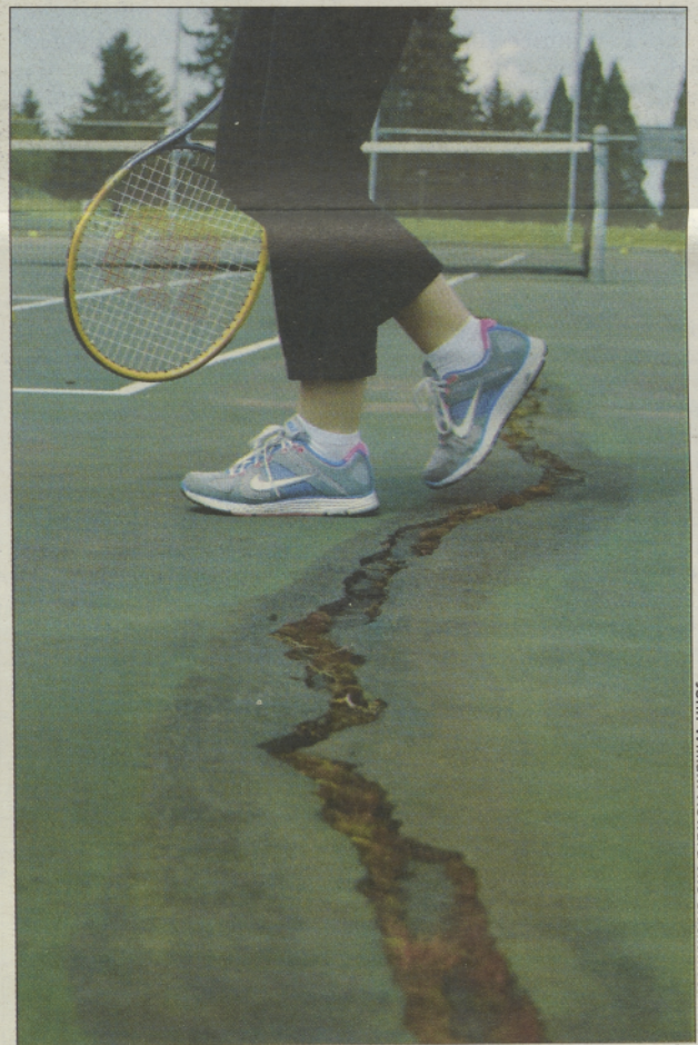
A tennis student walks across one of the many cracks in the aging courts. Cracks run not only across the courts themselves, but between each court, posing a danger to anyone who wishes to use them.
