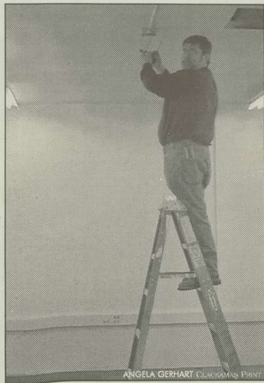
A worker wires lighting in one of three new spaces created in Barlow Hall. Originally one large L-shaped room, newly built walls create a general classroom, and two "flex lab" spaces to be used to house class computers and machines.
