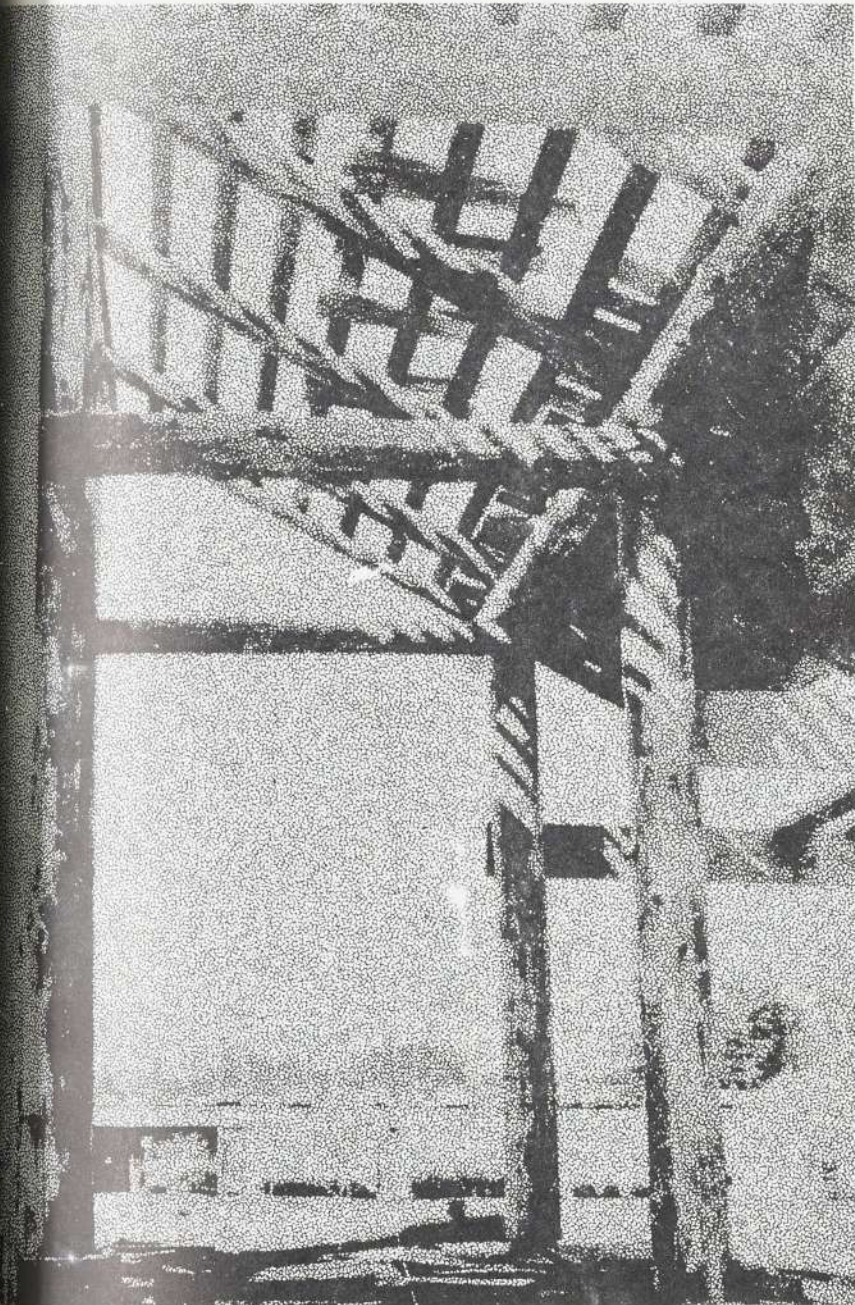
The spring sun casts cool shadows in CCC's new arboretum information center now under construction near Clairmont Hall. When finished, the center will provide information to the general public regarding the Arboretum/Ecology Pond on campus. (See story on page 3.)
