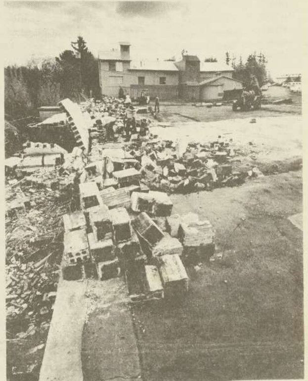
Clean up crews work on clearing away what remains of, Clackamas Community College's, Smuckers Hall.
