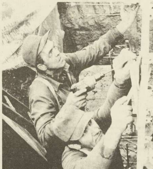
IN THE TRENCHES-- Construction workers Win Demenge (front) and Harold Walz prepare foundation for pouring of cement on Barlow Hall addition construction site. Contracted for $700,000, the new addition is expected to be completed sometime in April.
