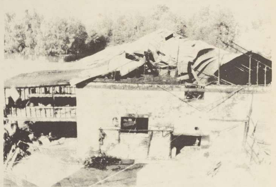
RUINED REMAINS--Smuckers building for $40,000 worth of damage to the College's displays damage with its caved-in roof and Art Center. The fire was also responsible
