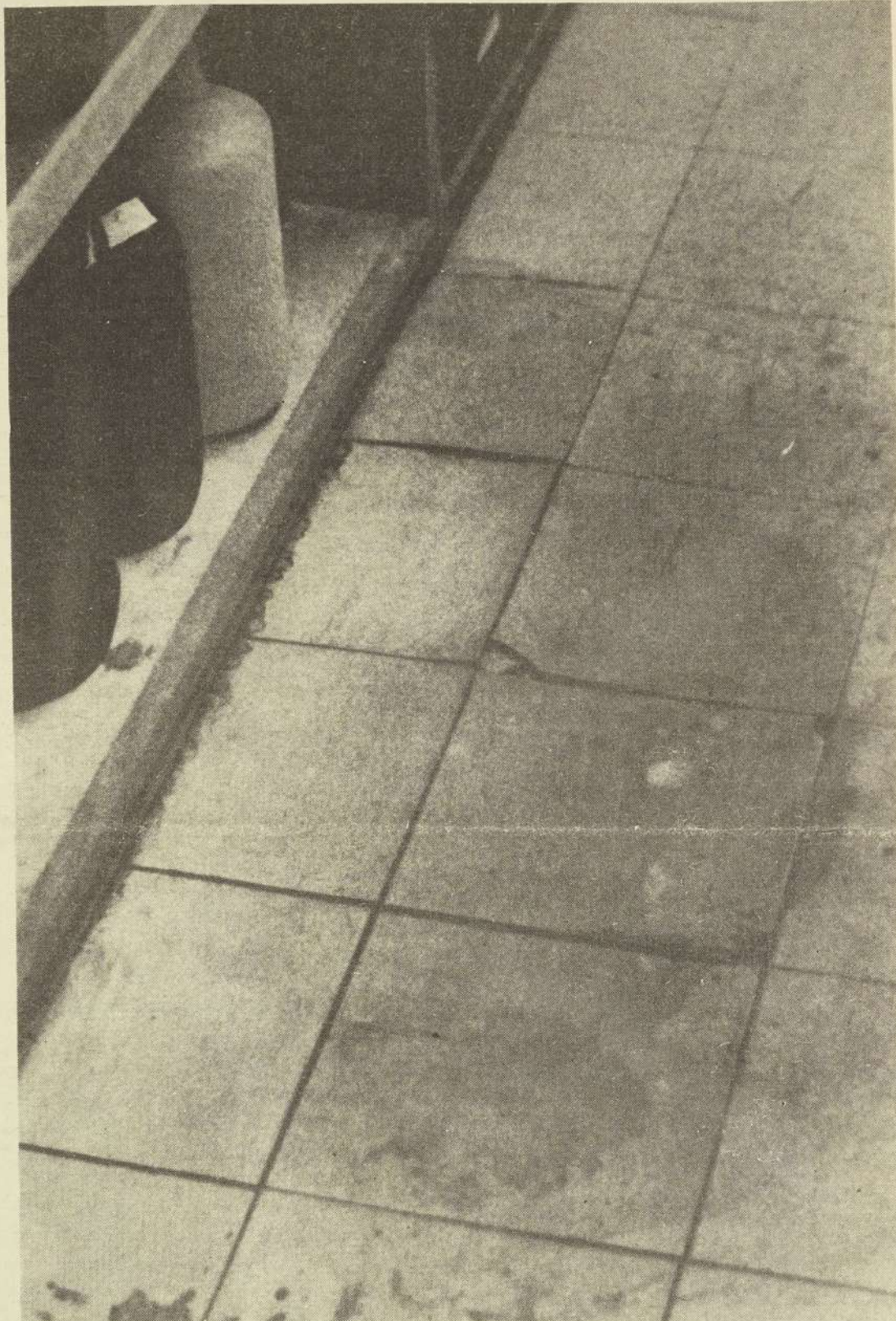
Loose tiles illustrate rotting floor conditions in outmoded science buildings. Passage of budget levy on April 4 will provide funds for new
