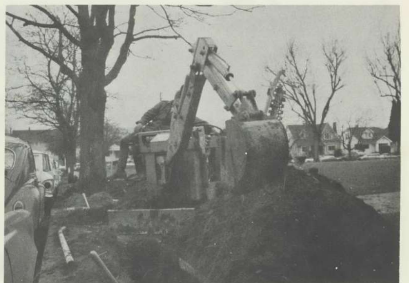
'Where's the ignition?' Members of the work crew of School District No. 1 prepare trenches for eventual installation of new street lights.
