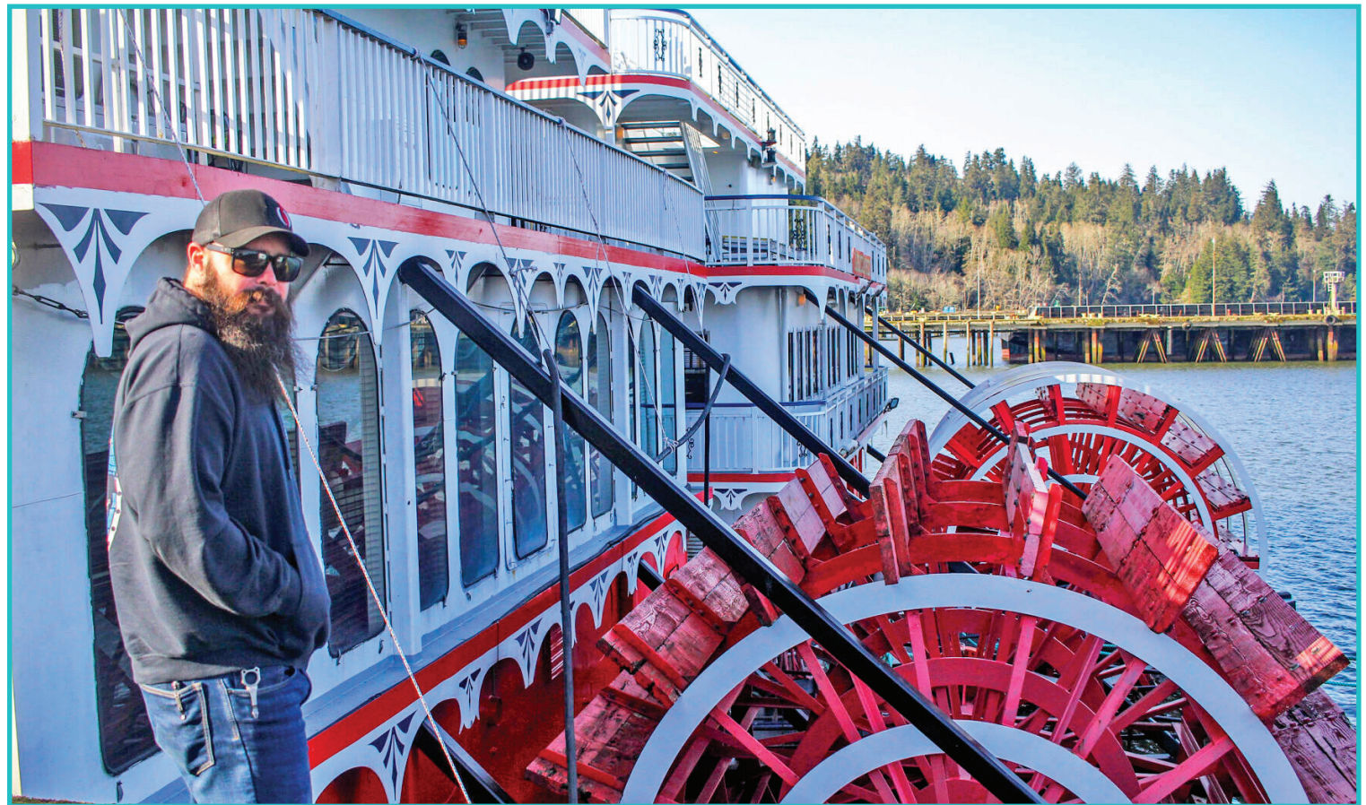
Kevin Sealy, in charge of bidding at WCT Marine & Construction, shows off the sternwheelers the company is repairing for American Cruise Lines at North Tongue Point.
