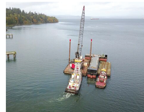
The Voyager leaving Tongue Point for the project at the Port of Kalama in 2019.
