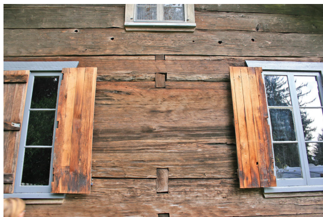
A single plank spans nearly the entire height of the windows.
