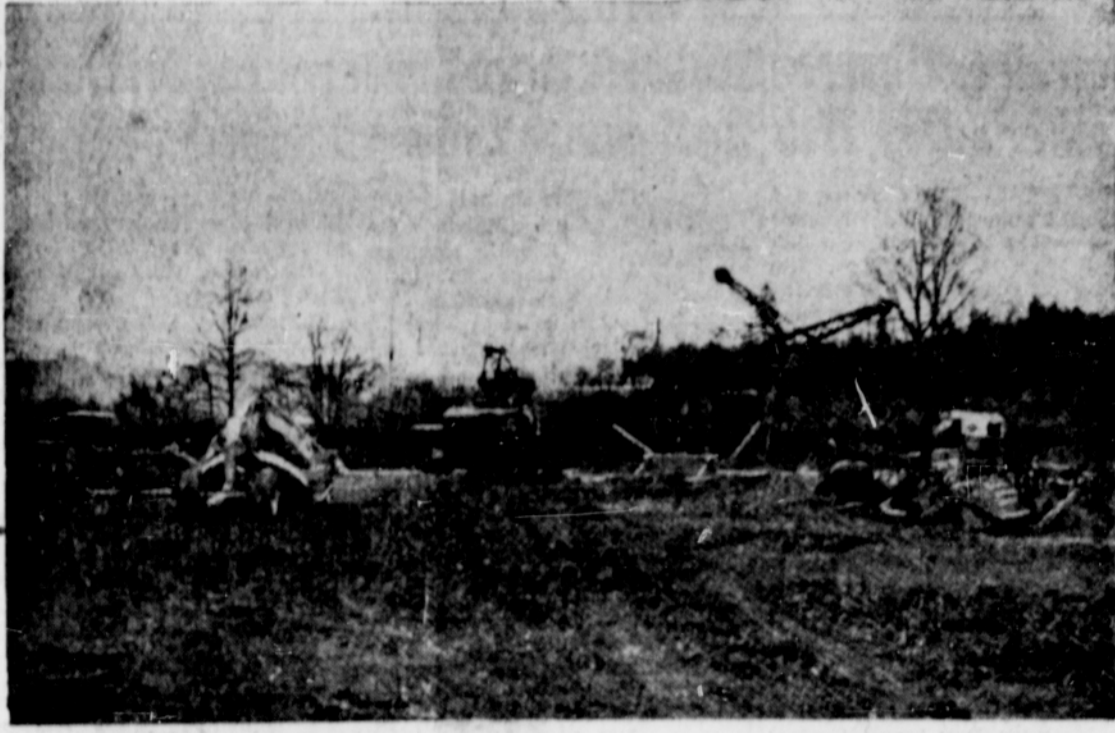
HEADQUARTERS of the McNutt Construction Co., contractor on the Highway Commission's Highway 99 relocation project north of Oakland, is shown in preliminary form. Work has just begun on this stretch of highway, while work is continuing on portions of the highway north of Drain and south of Canyonville. —Paul Jenkins picture, Roseburg News-Review.
