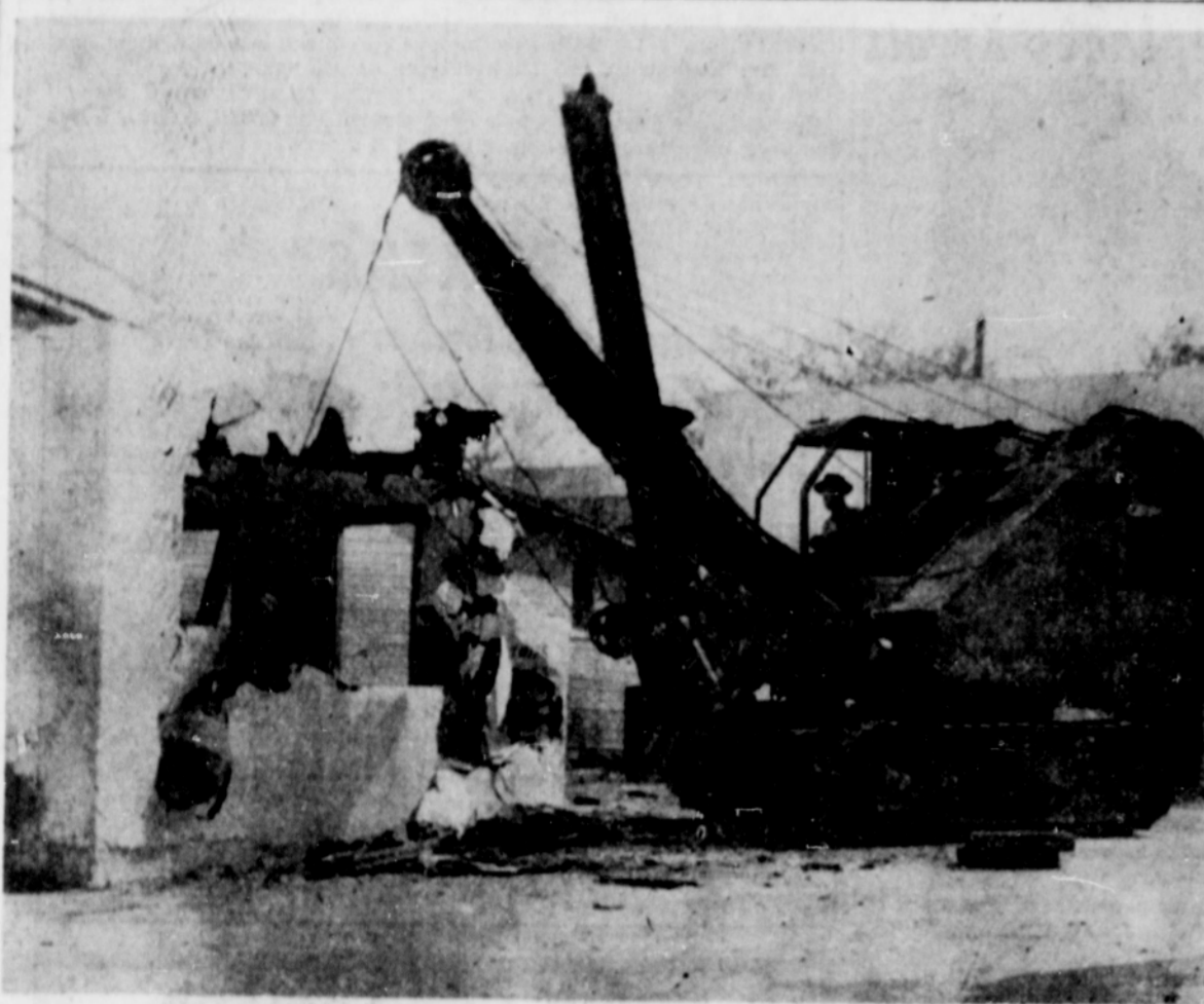
Portent of the times: wrecking of old Texaco station at 5th and Washington, once very busy when 5th street was the main highway, now torn down because of heavy traffic having shifted to Highway 99. The station is shown being wrecked by a 1500 pound ball swung on a crane by T. W. Busdrik. When company did not renew lease it had to have three buildings and all pavement removed. Lease read that the property had to be put back in same condition as it was before the station was built. Property belongs to Roy Short, probably will be leased for another business enterprise. J. S. Crepeau was contractor for the wrecking job.
