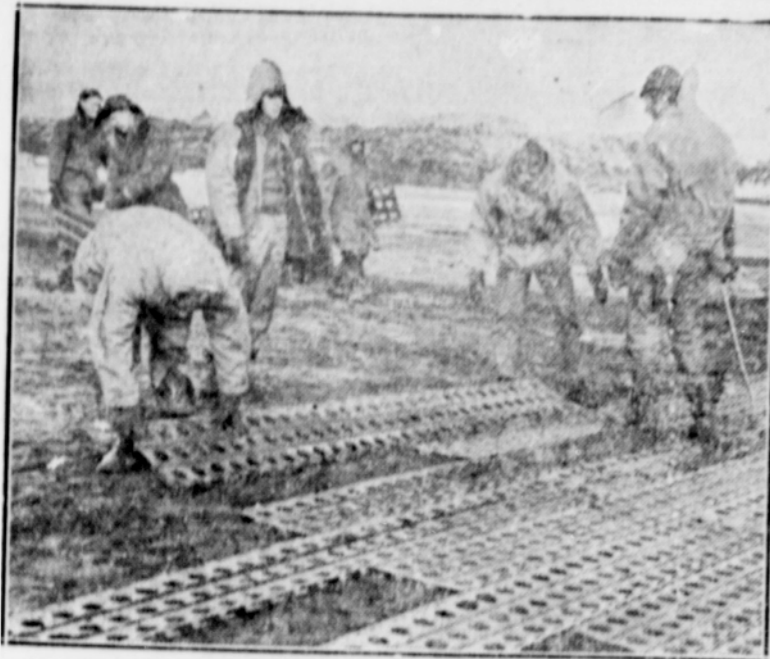
Bureau of Public Relations, U. S. War Department AVIATION ENGINEERS IN THE ARCTIC —A vital link in the chain of air bases built by U. S. Aviation Engineers in this landing field somewhere in the Aleutians. The field having been cleared, graded and rolled, portable steel landing plank is laid to complete the intricate system of runway and taxiways from which our aircraft will carry the war to the enemy.
