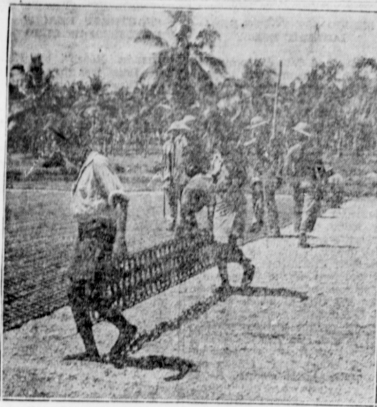
Bureau of Public Relations, U. S. War Department JUNGLE AIR FIELD IN SOUTHWEST PACIFIC —Utilizing native materials and labor, U. S. Aviation Engineers have carved a mile-long runway out of the heart of the jungle. Natives are shown laying the portable steel landing mat under the direction of the engineers. The foundation is a bed of crushed coral which is locally available in plentiful quantities.
