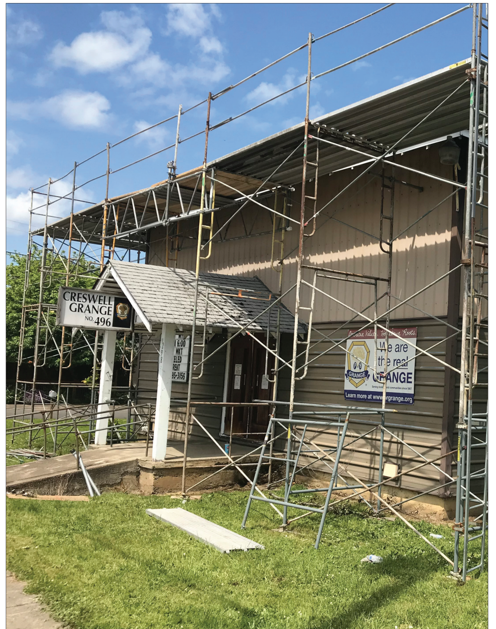
The real Creswell Grange is surrounded in scaffolding Tuesday, May 5. Crews are repairing and fortifying the roof, which was damaged during last year's snowstorm. During the pandemic, the Grange has been asked to close. When it's able to open again, meetings are the second Monday of every month. The potluck starts at 6 p.m. and the meeting begins at 7 p.m. STAFF PHOTO
